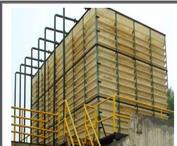
Natural Cooling Towers
