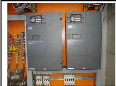
VFD in air washers
